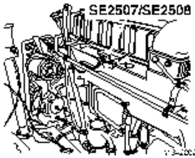
Figure 6 SE2507 (PID !05)/SE2508 (PID 102) Charge air temperature/pressure
